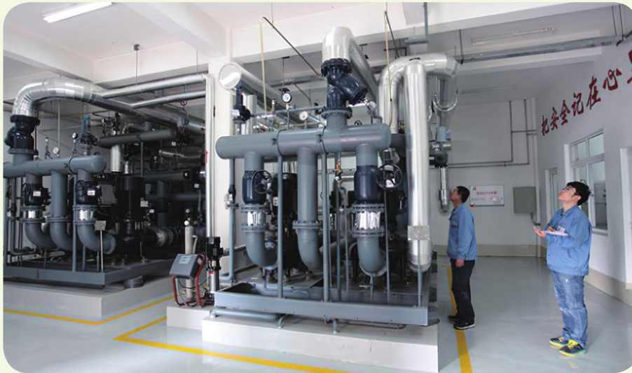
▲ Central Heating Facilities of Qingdao Energy Group
